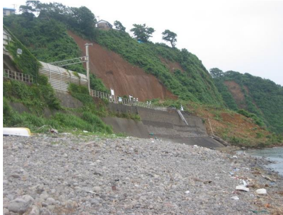
Fig. 2. Omigawa landslide triggered by the 2007 Chuetsu Oki earthquake, Japan. The landslide mass was formed in weathered sandstone on a steep slope of 55-60°.
